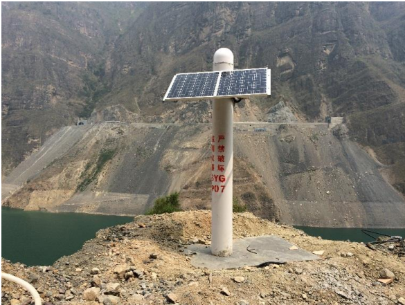
Fig 1. Observation site near landslide area
